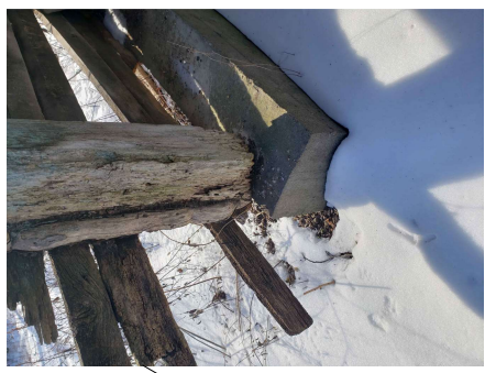
REPLACE WOOD POST
