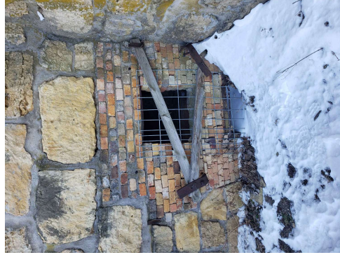
BRICK IS IN GOOD CONDITION — REPLACE GRATES AND REMOVE PROTRUDING STEEL
