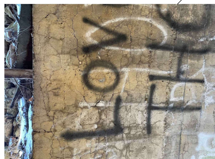
SEVERE CRACKING THROUGHOUT WALL
