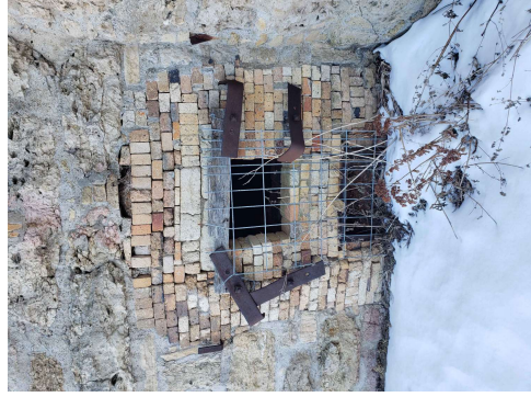
BRICK IS IN POOR CONDITION — REPLACE GRATES, BRICKS AND REMOVE PROTRUDING STEEL
