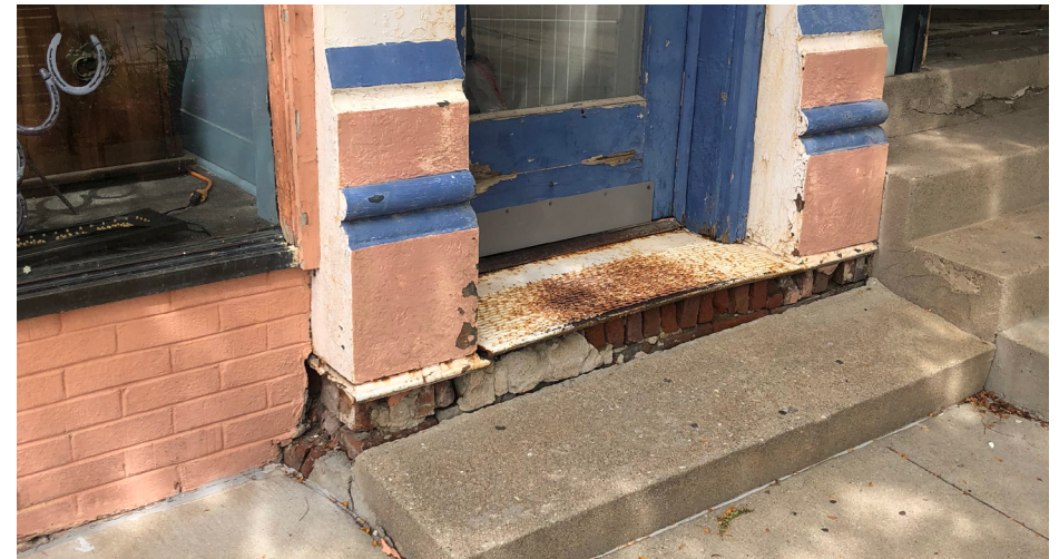
Figure 19: Deteriorating part of a building
