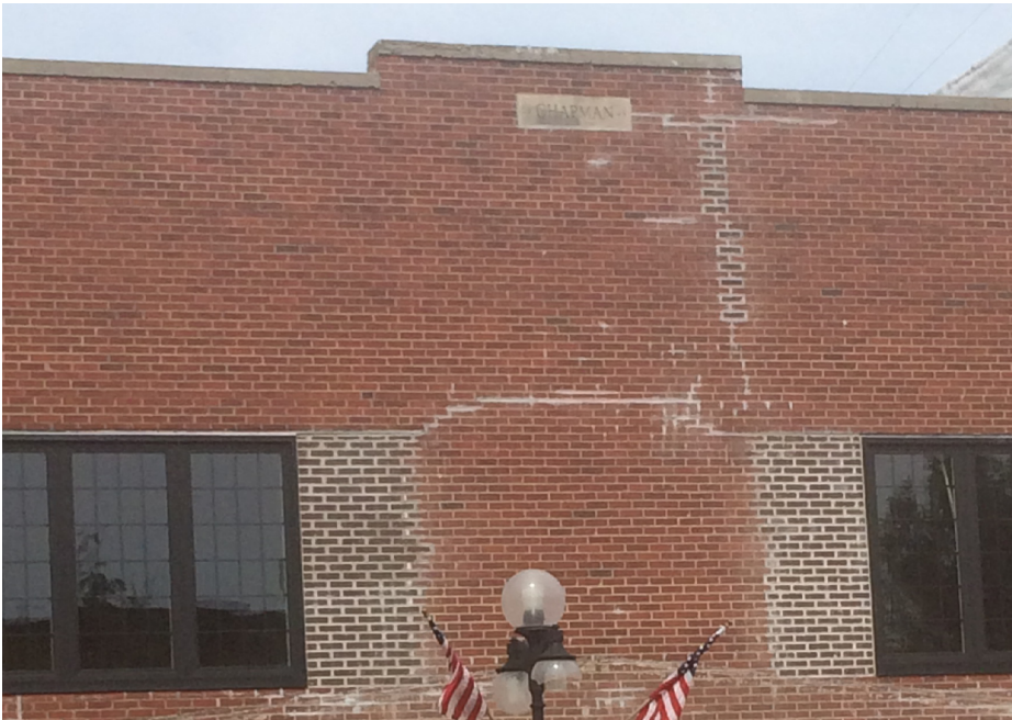
Figure 17: Storefront showing lateral joint failure on brickwork
