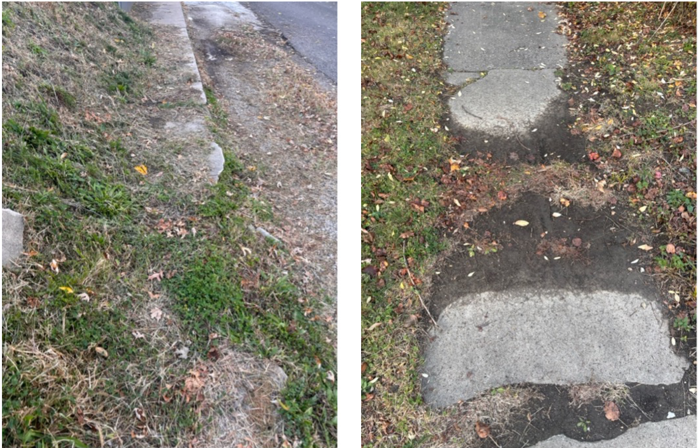
Figure 11: Sidewalk conditions on Garnet St (Left) and N Central Avenue (right)
