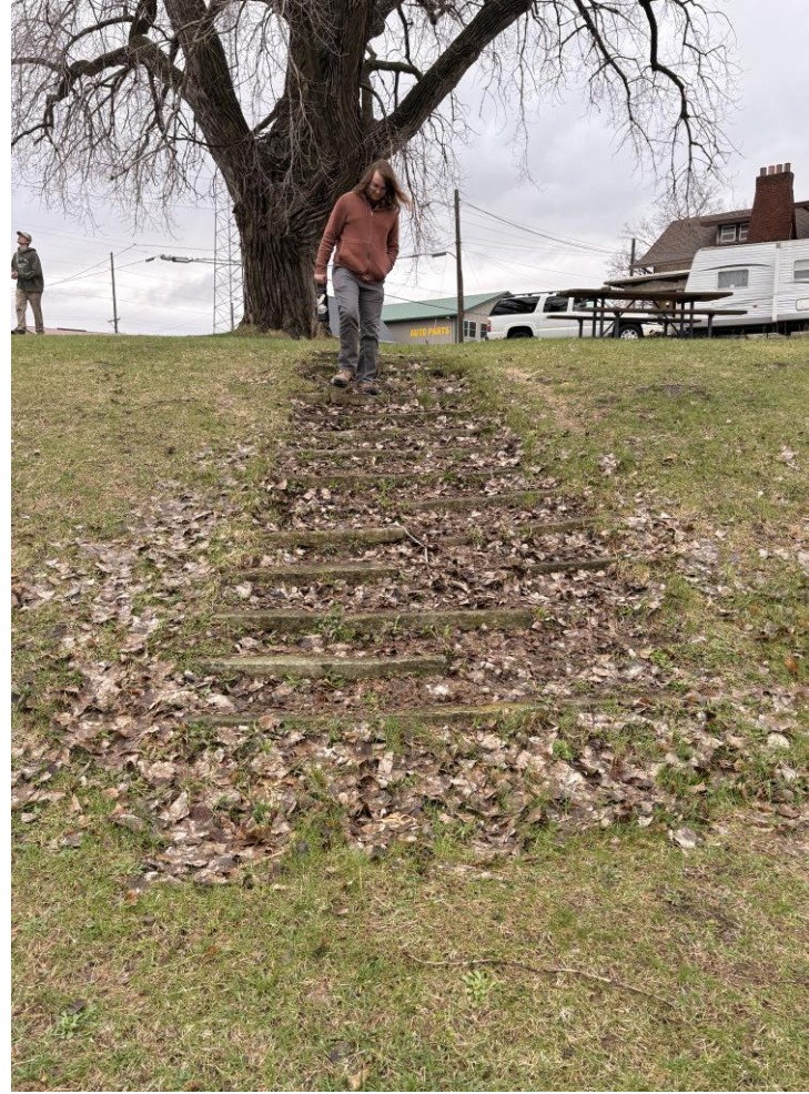
Stairs down to lower level in disrepair
