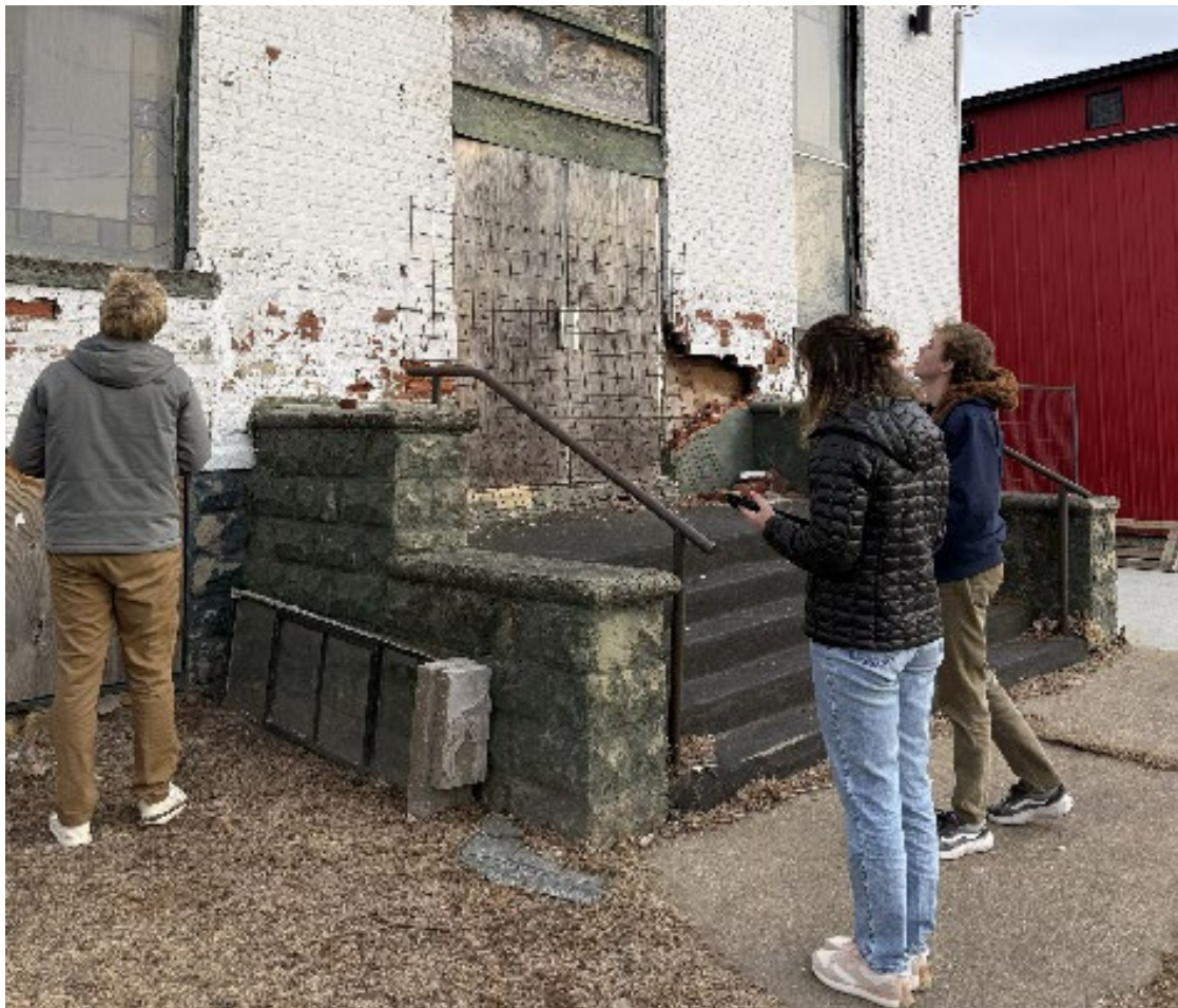
Figure 1. Entrance of Bethel showing brick columns to be replicated
