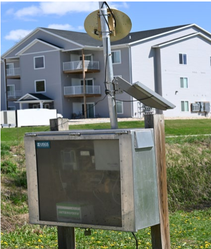
Figure 8.3 ream Gauge Monitoring Station on Wapsi Creek
